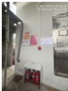
Fire-extinguishers at the frozen warehouse.jpeg
