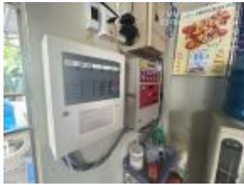
Fire alarm control Panels.jpeg
